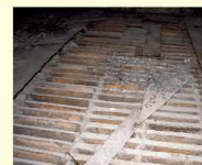
Section of kiln floor showing the long 'kiln-bricks' resting on the arch supports.
